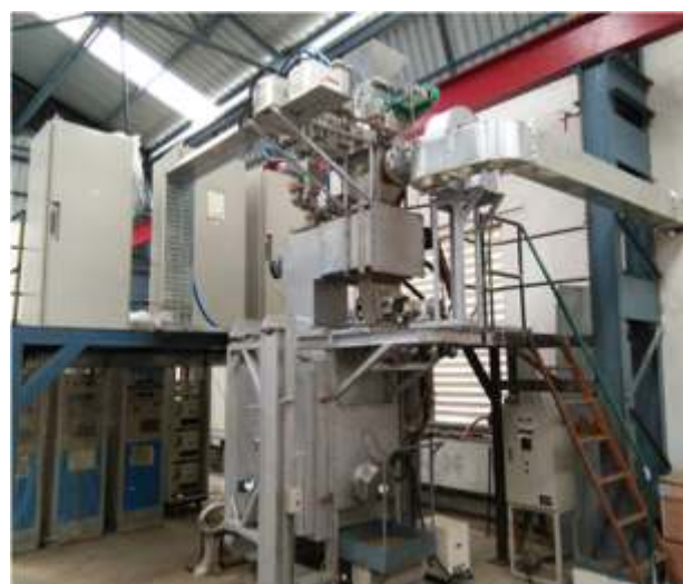
Fig. 3: Microwave assisted prototype plant installed at PML
